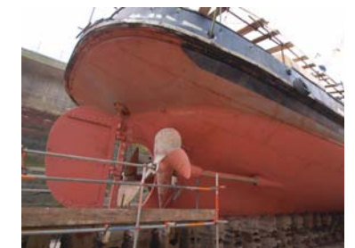
Scaffolding rigged ready for the removal of the props which took some coaxing and the use of a 60 ton jack.
