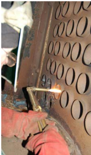
Boiler tubes being burned out by NSL's best Boiler Man – Jimmy Ash
