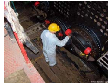
The boiler front after 'oiling' (Volunteer John Pickering adds the final touches)
